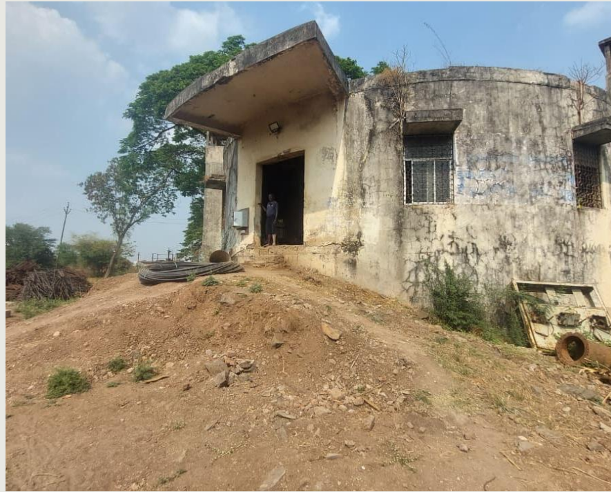
Old STP pumping station got submerged and broke down
